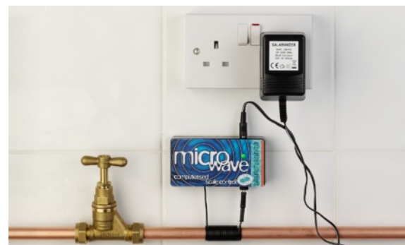
Microwave in situ
